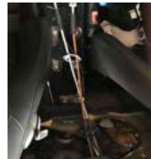
The cables going through the firewall (looking down).
